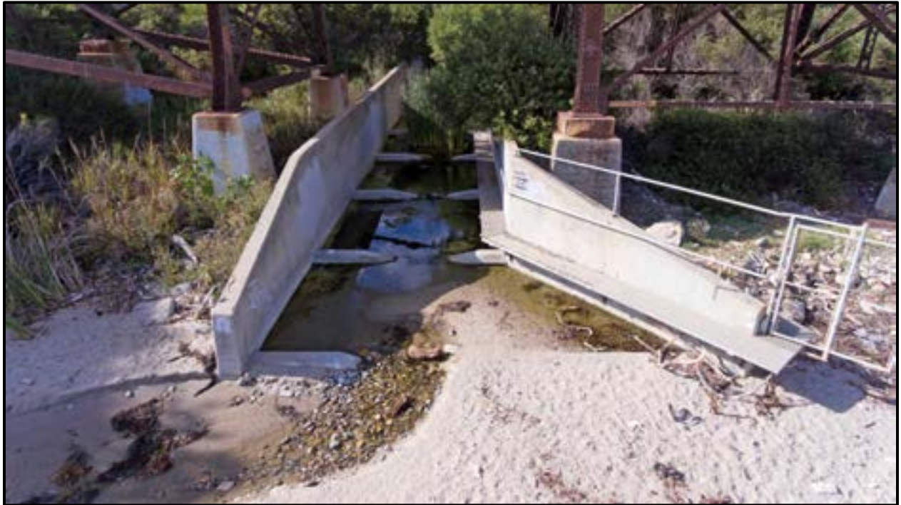
Figure 4-13. Sediment accumulation and vegetation growth in the Arroyo Hondo Creek culvert in Santa Barbara County 2017. This culvert ends at the beach similar to Solstice Creek.
