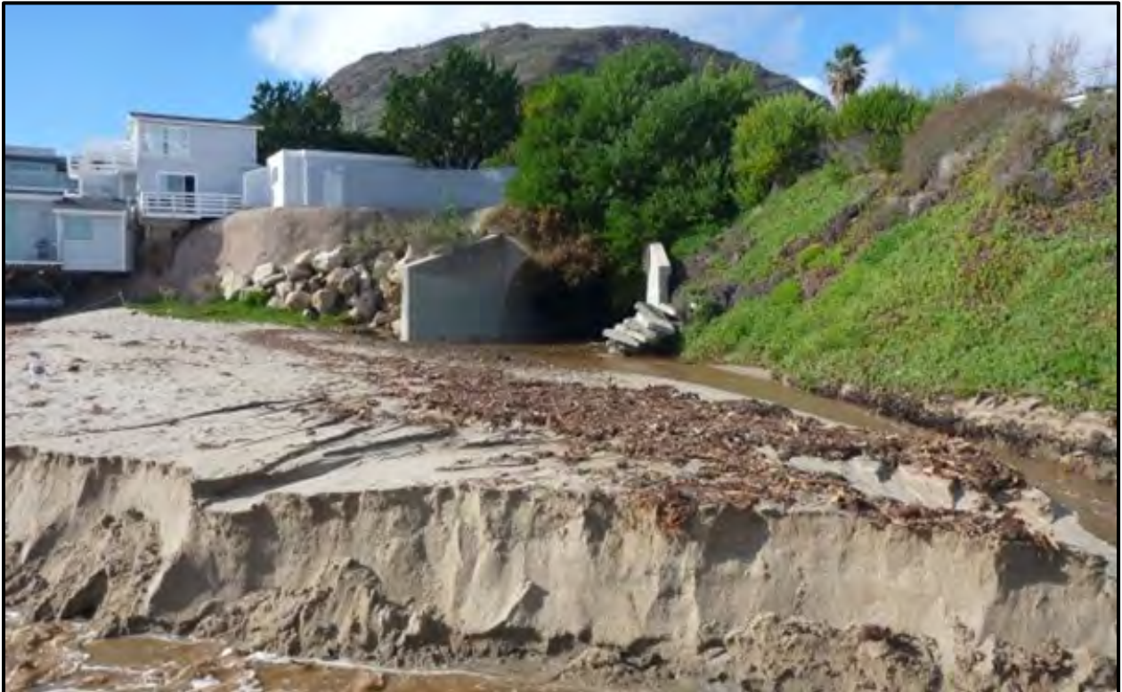
Figure 6-1. Solstice Creek (unknown date). After exiting the culvert, the creek took a sharp left turn, followed the base of the highway embankment, and then took a sharp right turn towards the ocean.
