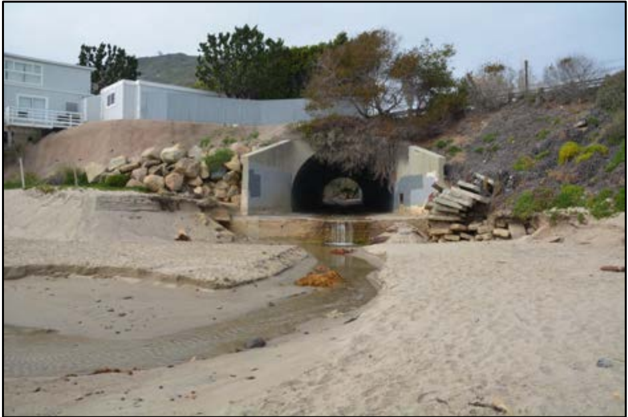
Figure 1-3. Looking upstream towards Solstice Creek Culvert, February 2, 2017. Following storms in late January, there was a four-foot drop at the culvert outlet.
