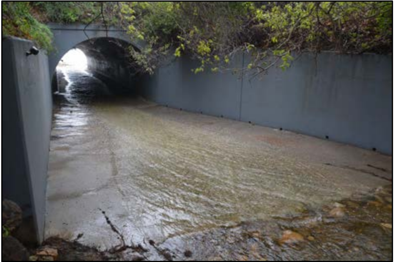
Figure 3-10. Highway 1 Culvert on Solstice Creek, February 21, 2017. No sediment deposits were observed in the culvert. Flow conditions in the culvert would be too shallow for passage.
